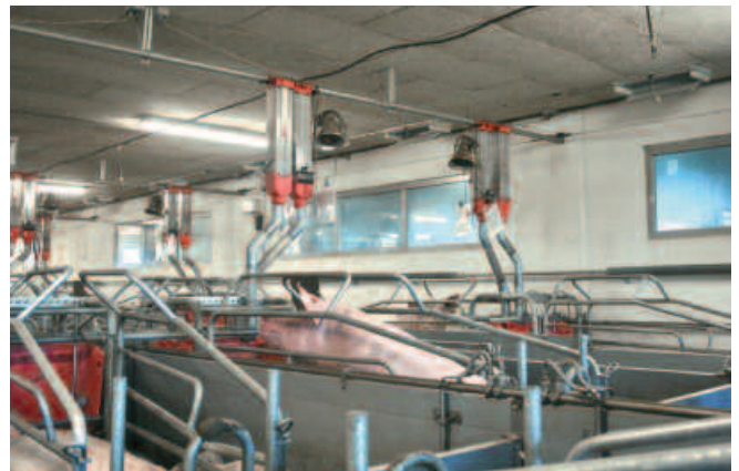
Building C with the IL inlets mounted in the ceiling along the wall.
