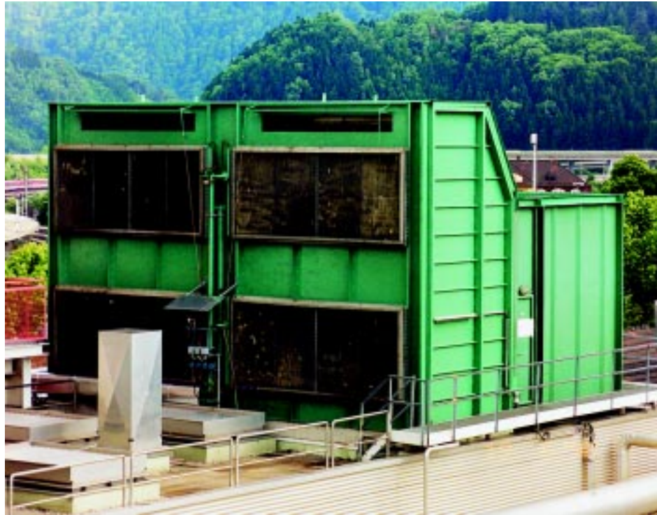
The modified filter house with a built-in Munters PreCooler.
