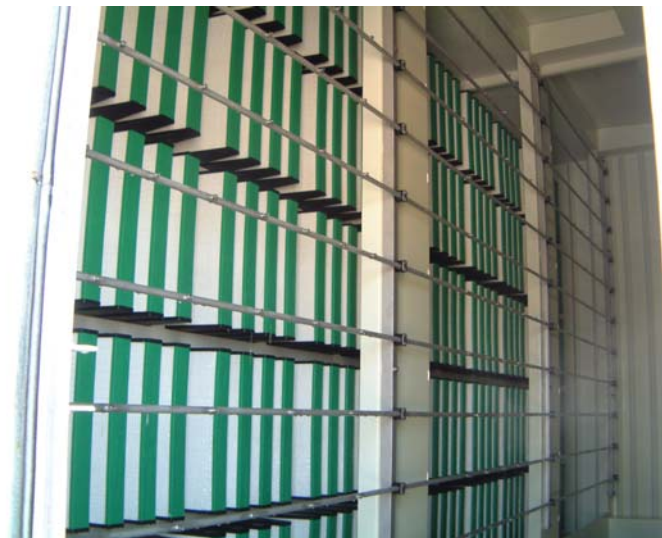
Installed fogging arrays in air intake
