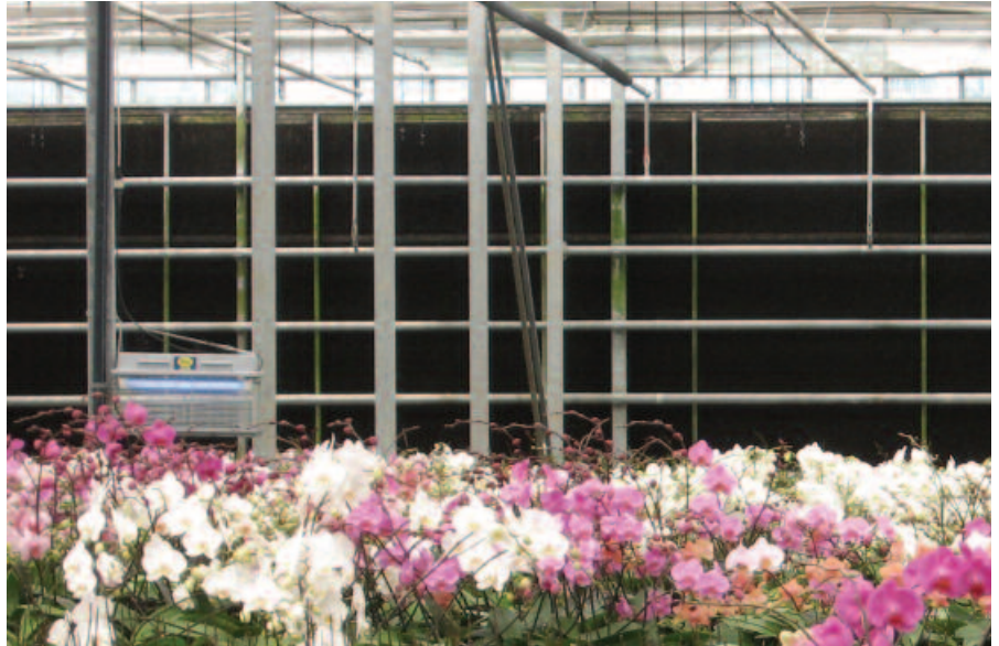
The wall of CELdek® evaporative cooling pads.
