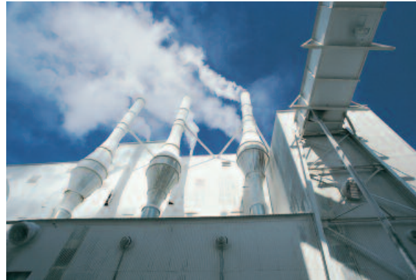
Stack rain separation units help to clean the emissions.
